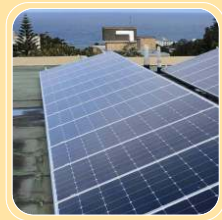
SOLAR POWER (COMMON)
